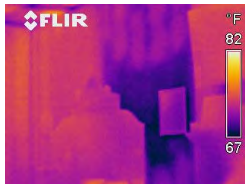
Figure 2a. Thermal image of missing insulation
