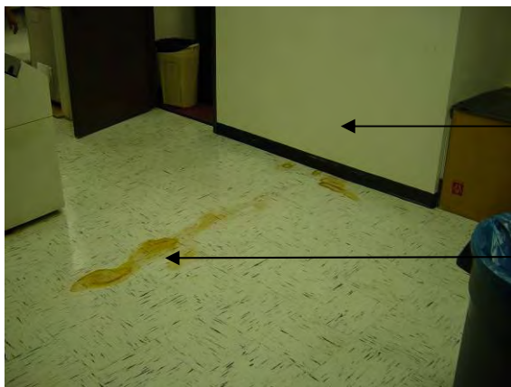
Figure 7a. Stains on the floor.
