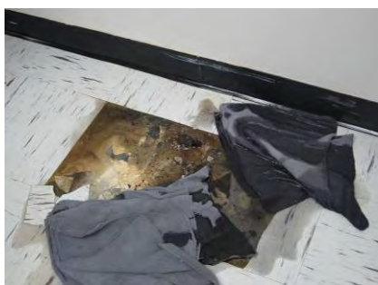
Figure 8a. Leak found.
