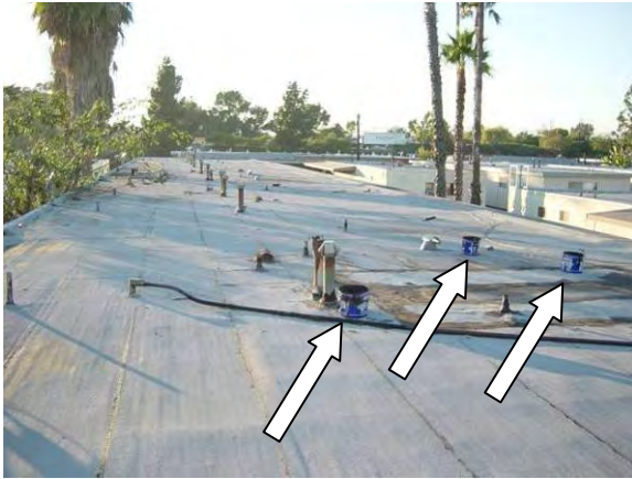
Figure 3. Roof with problem spots.
