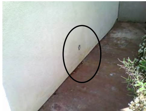
Figure 10a. Visual of sewer cleanout leak.
