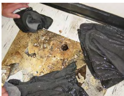
Figure 8b. Hole uncovered.
