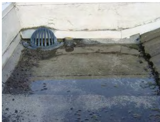
Figure 5b. Improperly installed drain allowing moisture intrusion.
