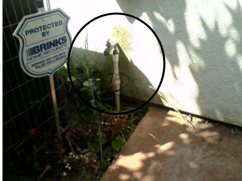
Figure 9a. Visual of pipe leak at stucco wall.
